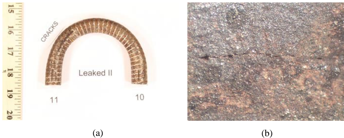
Figure 2: (a) The bend tube after removal of fins and (b) SCC on the apex of u ben sample/
